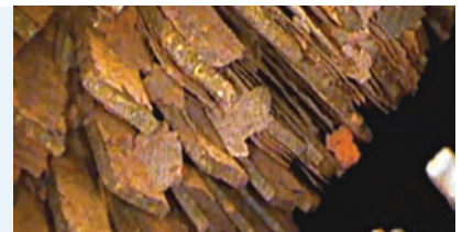
Before. Impacted deposits on finned tubes.
