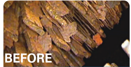
Impacted deposits on finned tubes
