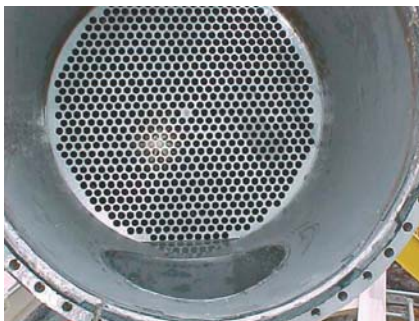
Top photo: A heat exchanger tube sheet before water blast cleaning. Bottom photo: The same heat exchanger tube sheet after cleaning.
