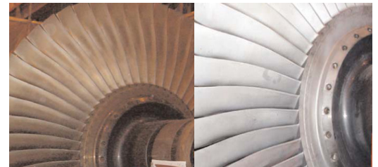
Turbine before & after
